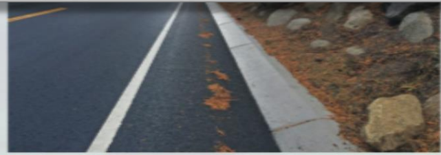
Rock slope stabilization and gutter pans added to sections of Highway 89 between Meeks Bay and Emerald Bay
